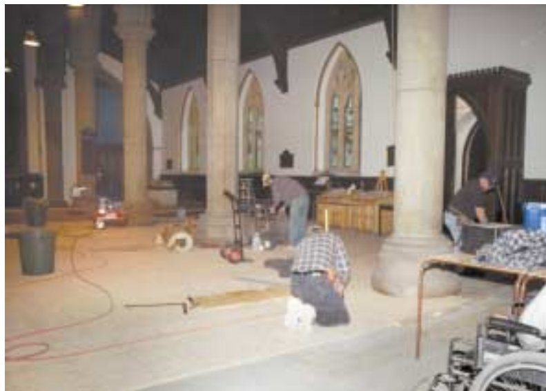
Refinishing and minor repairs turned into a whole new floor. Without the pews, the nave was wide-open.
