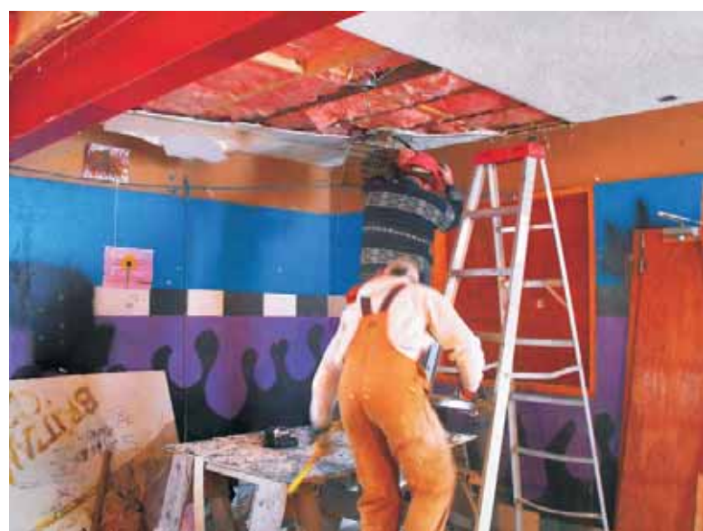
Construction workers began to dismantle the old staff-house in mid-January. A new administration and staff building that completes the refurbishment of the camp will be ready for the 2010 camping season.
